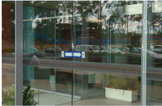
Accessible Entrances and interior doorways (automatic doors with safety markings on glass).
